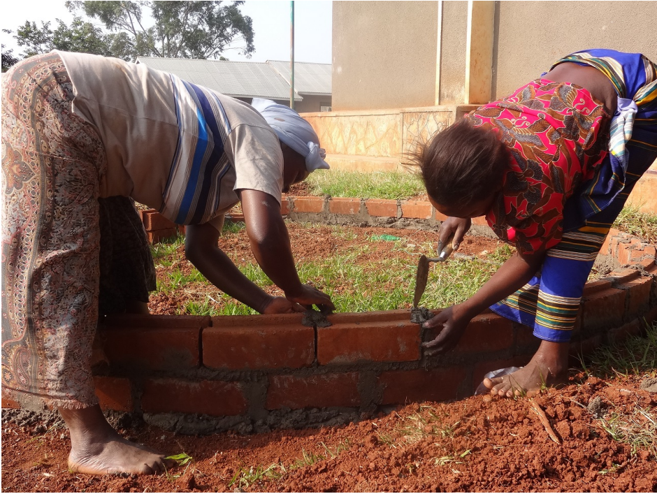
KWDT trained ISSB masons; Betty Kajuule and Rose Namukasa to construct bigger rainwater harvesting tanks appropriate for communal places e.g. schools at Kojja S.S.S
