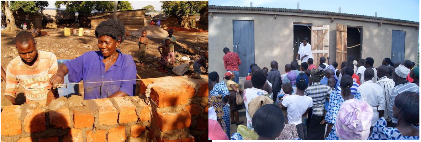
Lydia Kateregga, the only EcoSan female mason, demonstrates the proper use of the EcoSan toilet upon its completion, in Buleebi landing site.
